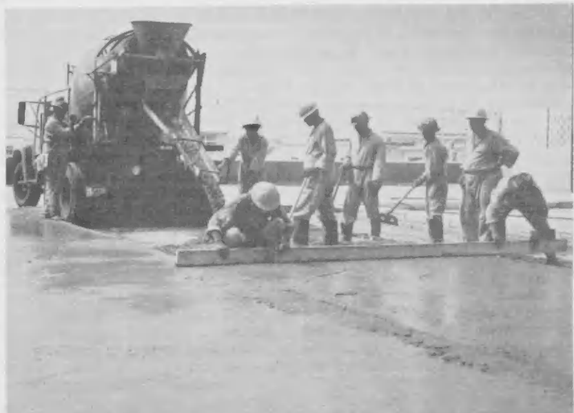
TO LEVEL the concrete, masons extend a board from one screed to another and move the concrete before them leveling and filling the area. PA NIVELA e concreto, metselaarnan ta pone un pida palo for di un lata pa otro y ta move e concreto cu e palo, asina nivelando y yenando.
